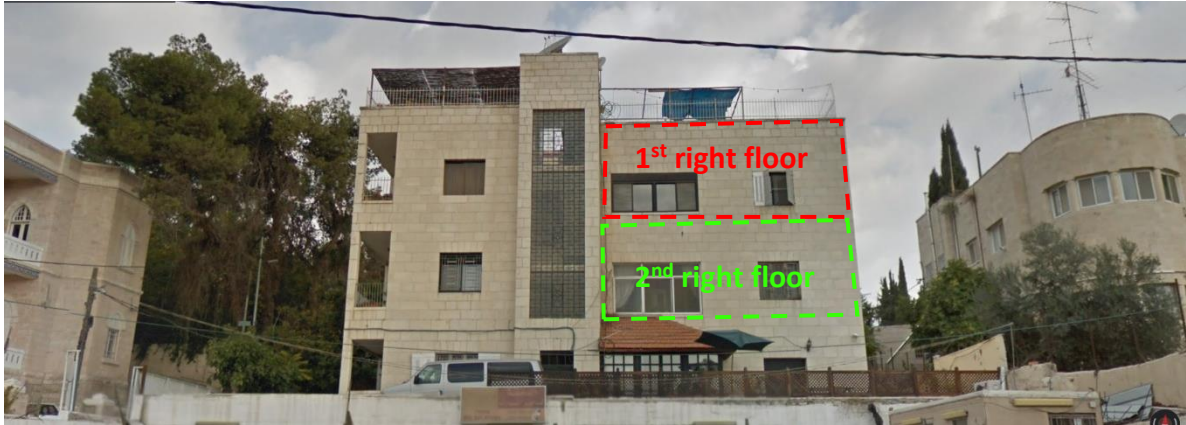
Photo of the building and location of the apartment of the first floor where the works are taking place
