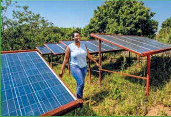
In Manica province (Mozambique), Donna Isabel Vilanculos's lychee farm is irrigated through a solar pumping installation. © Enabel - Isabel Corthier
