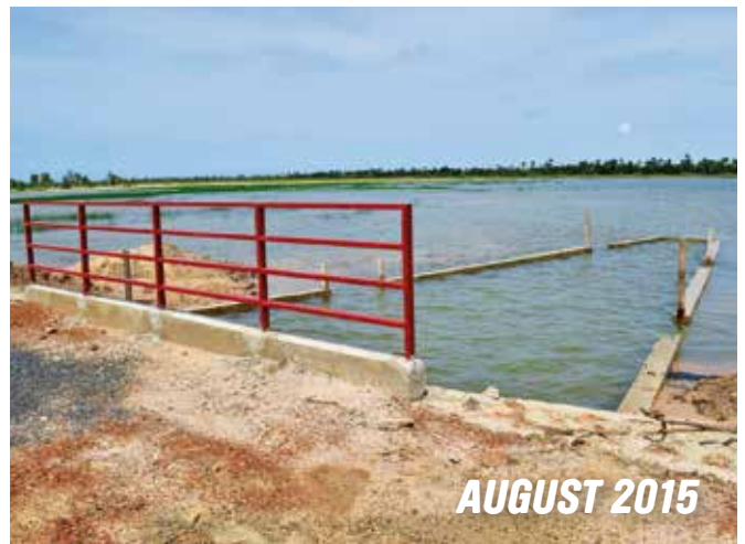
The Bakhala Valley (Fatick) during the dry and during the rainy season. Above, one of the three anti-salt dams built by BARFAVOR in response to the demand of the people of Bakhala. Photo: © BTC / Marcella Pasotti
