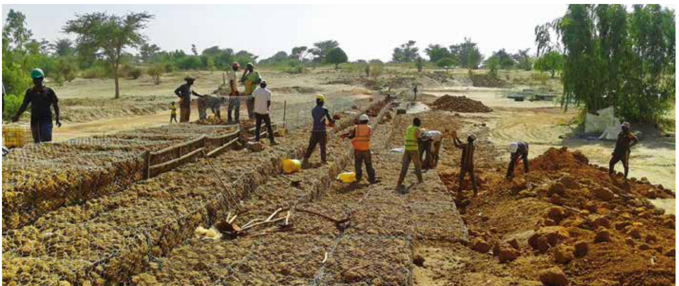
Construction site at Notto Ndioukhane (Thiès), construction of a filtering embankment. Photo: © BTC / Nicolas Widmer
